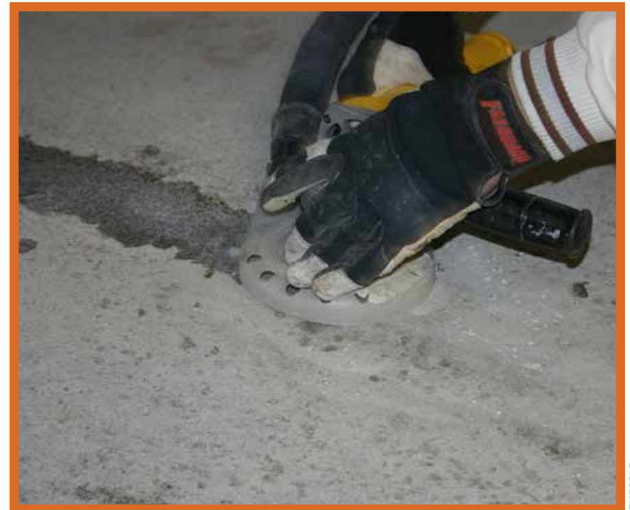
Thorough crack repair and efficient grinding are becoming commonplace prior to installing an overlay.
