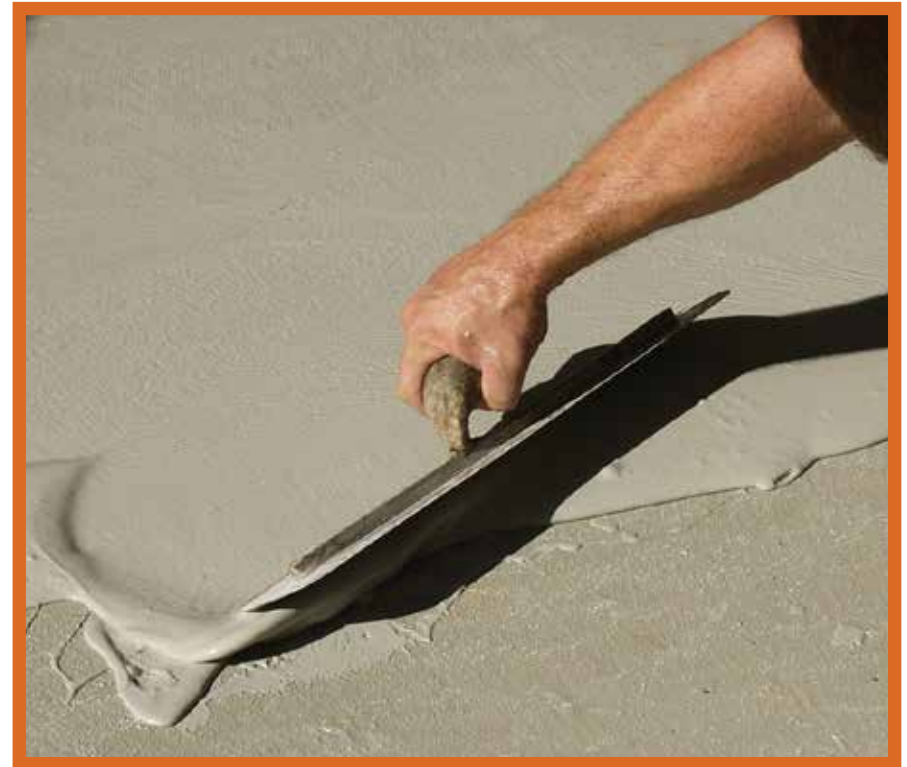
The design community likes the clean look, without any grout lines, that microtoppings can provide.
