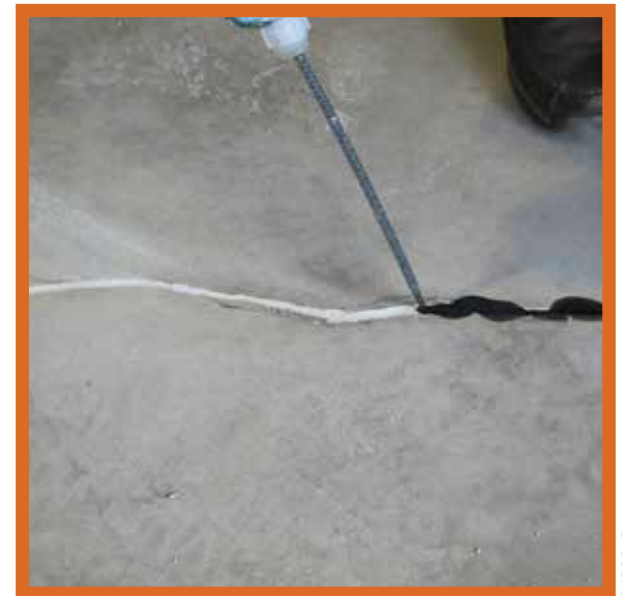
Epoxy crack fillers are popular for repairing cracks prior to overlay installation.
